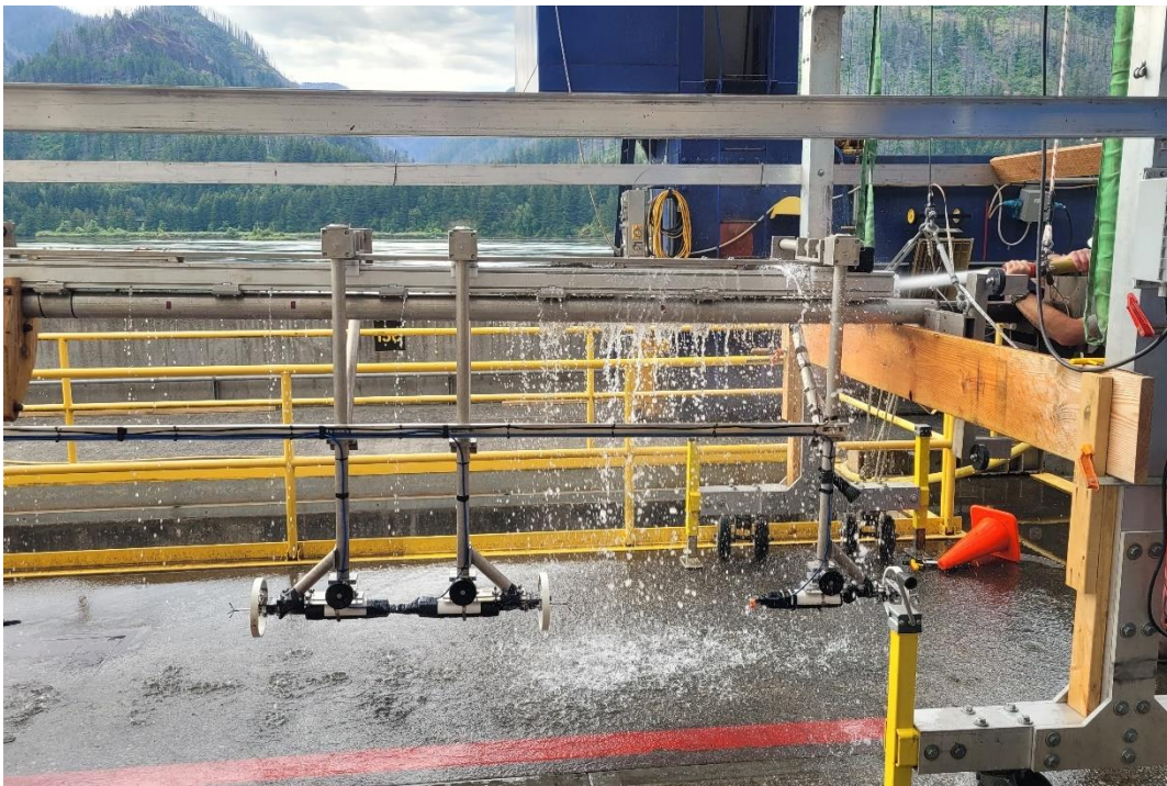
Photo 3-5 Flushing of Grit from Traversing Beam (Side View)
