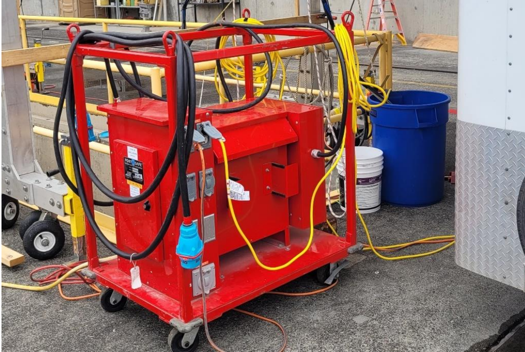
Photo 2-17 Load Center used to Power Data Collection Equipment
